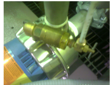
Check Valve and Connection
